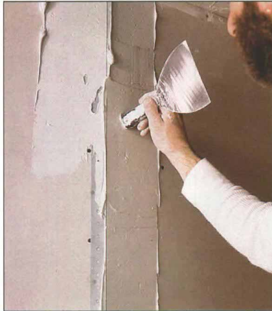
Recessing lumps. Lumps are easily taken care of with a knife handle. But don't use setting-type compound in a nail hole: It dries so hard that it's difficult to sand.
