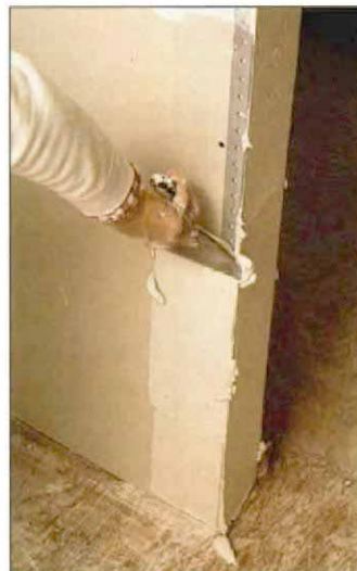
Outside corners. Straight outside corners get covered with a metal corner bead, a layer of setting compound and two coats of all-purpose compound. The corner bead helps guide the tapping knife.
