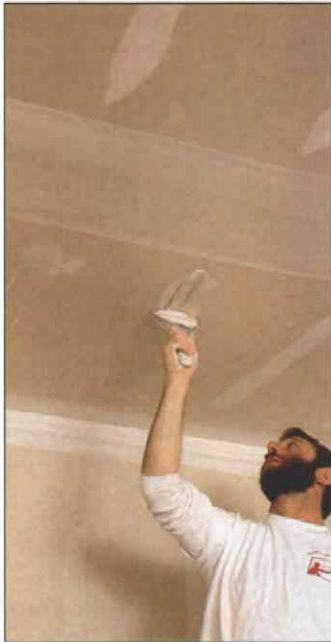
Spotting nails. Nail holes get filled with repetitive coats of ready-mix joint compound.
