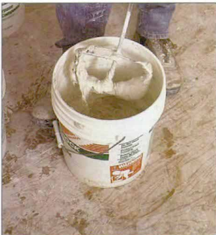
Mixing mud. Powdered, setting-type joint compounds are mixed with water. A mixing paddle and a 1/2-in. drill come in handy for stirring up large batches.
