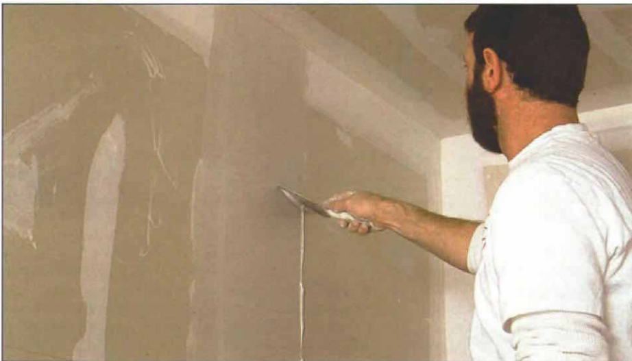
Doubling a joint. Butt seams are high points on the drywall's surface. One way to make them less conspicuous is to spread a band of compound on either side of the seam, then go over the center after the bands have dried. In this photo, Henderson has just gone over the center of the seam with a troweled layer and is now feathering the edges.
