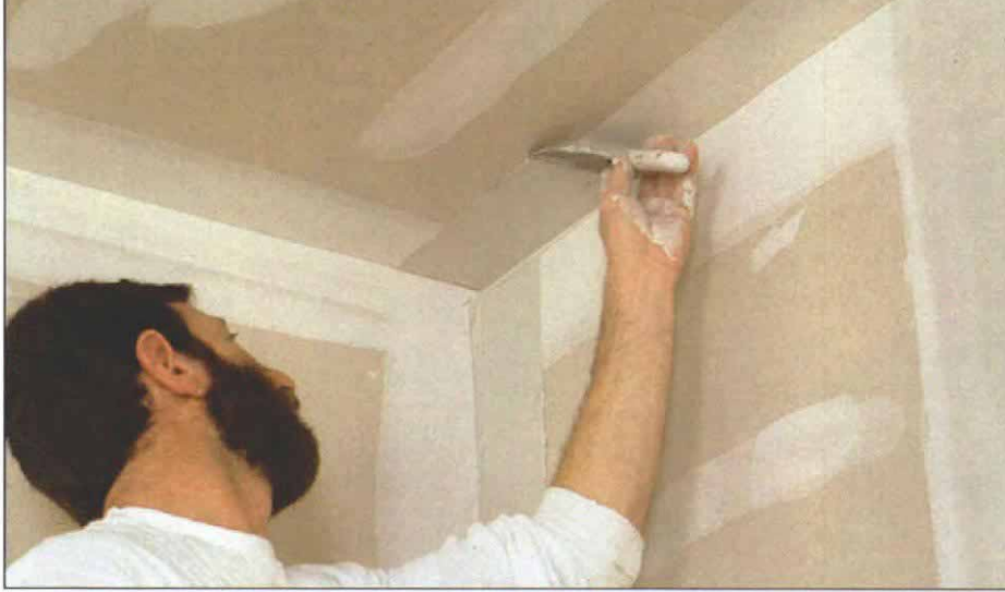
One side at a time. Inside corners are finished by coating one side, then doing the second after the first has dried. Inside corners only need one finish coat instead of two, so the waiting time doesn't slow down the schedule.
