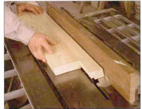
Cutting the siding groove. A dado blade cuts a ½-in. by ½-in. groove in the windowsill to accept the siding.
