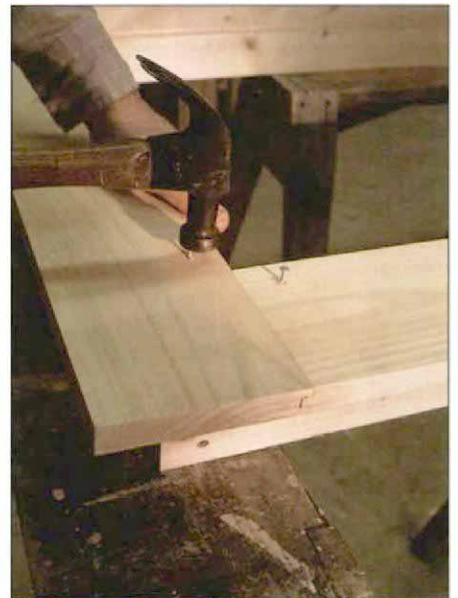
Nailing on the casing. Pilot holes are drilled for 6d galvanized nails. The mortise-and-tenon joint that joins the head and side casings provides weather resistance at the joint.
