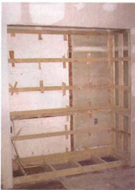
The opening. New studs frame the sides, but the back wall of this former closet was straightened with 1x3s and shims.
