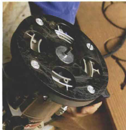
Making the brackets. Over a hundred pieces went into the brackets and modillions, making their fabrication perfect for template routing. In the photo to die right, the author routs the profile of an outer lamination. The next pass, with a \frac{1}{4} -in. bit and collet (above) will mill the fretwork pattern in its face.
