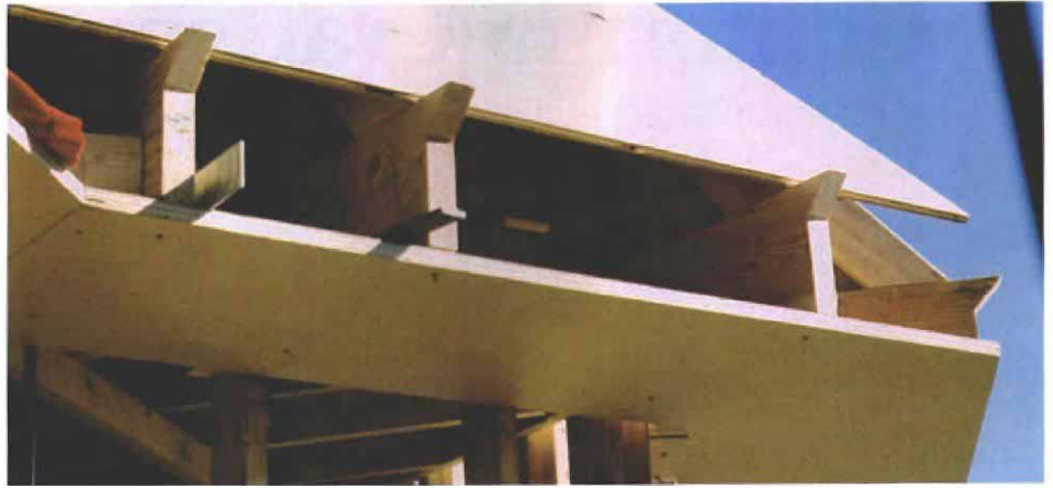
Supporting the main cornice. Triangular trusses made of Douglas-fir 2x6s fan out from the wall framing to serve as backing for the cornice roof and soffit. The trusses are held in the same plane by plywood gussets. The beaks on the bottom cords of the trusses anchor the crown molding.
