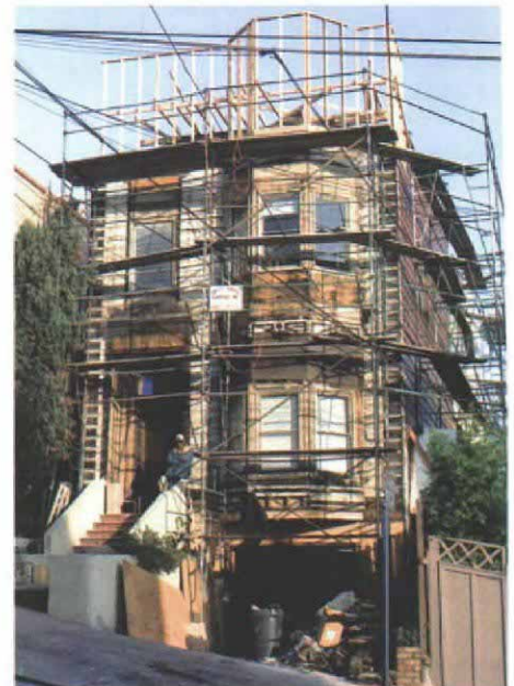
Putting it back. Guided by an old photo of the house, the author extended the parapet and the bay window to their original heights, then began work on the restored cornice (top).
