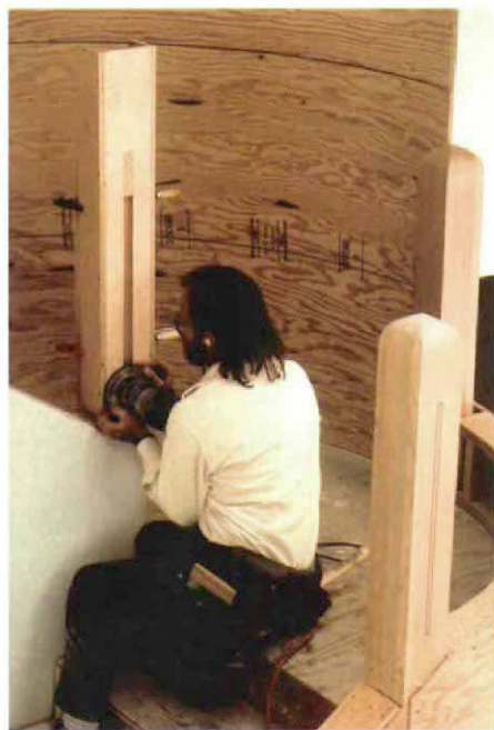
Detailing the posts. A simple U-shaped plywood box that fits around each square newel post served as a template to guide the router as it cut the vertical details of the newels.
