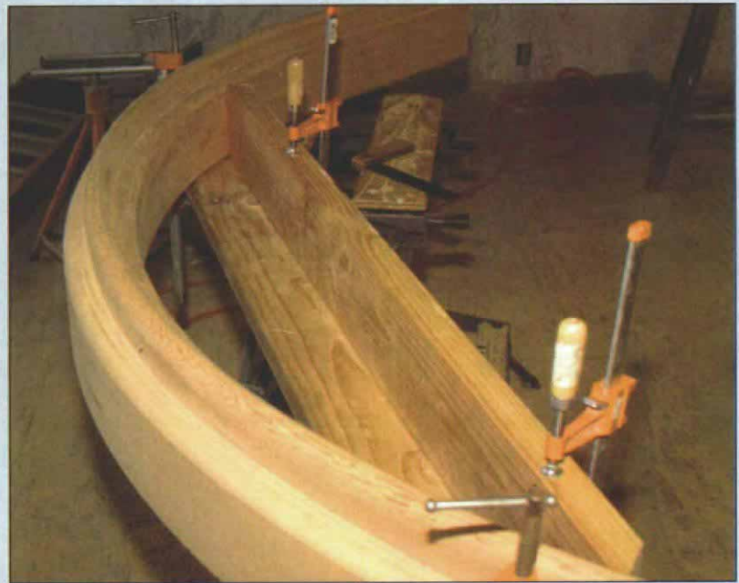
Cutting the curved handrail. A straight jig made of 2x8s enabled the author to find the length and the angles for the curved handrail. After the length and the angles were determined, the handrail was clamped to the jig, and it was used as makeshift miter box.
