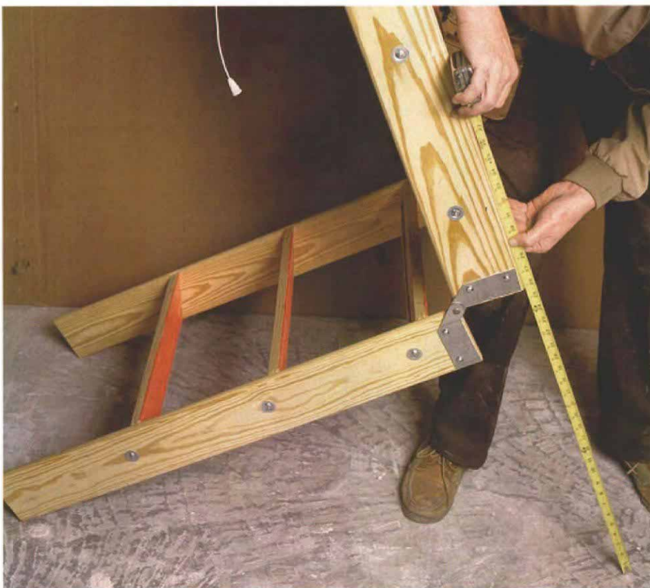
Measuring for trimming. With the bottom section folded under the middle section, the author puts his weight against the stairway to ensure it is fully extended. He measures along both the top and bottom edges of the stairway, transcribes his measurements on the bottom section, connects the dots and makes his cut. The trap door's pull cord can be seen hanging in the top of the photo.
