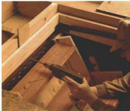
An extra screw for insurance. A third mounting screw in a folding stairway's piano hinge strengthens the installation. The author drills through the hinge and the jamb and into the rough framing. The large spring at the top of the photo is one of a pair that holds the stairway and its trap door closed to the ceiling.
