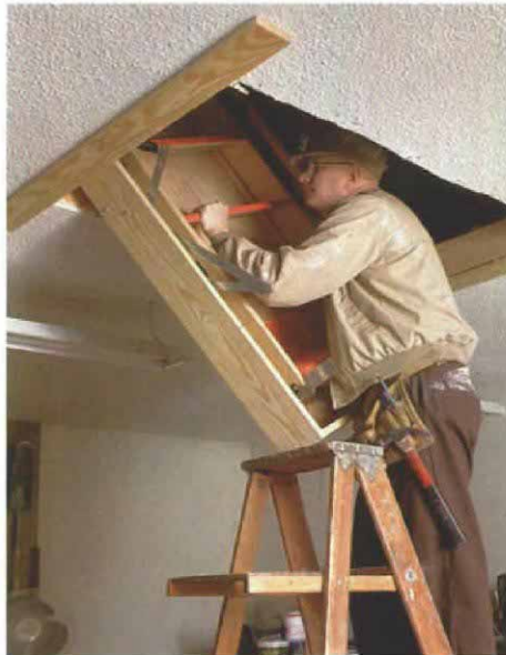
Support during installation. Ledgers screwed to the ceiling provide temporary support for the stairway while the author shims and screws the frame to the rough opening.
