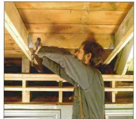
Metal hangers for a strong connection. Because the header is supporting part of the roof load, the author uses a double 2x on edge and connects the header to adjacent rafters with metal hangers.
