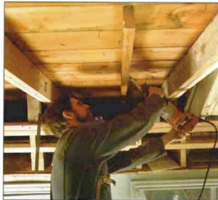
Make way for a skylight. If a skylight can't fit between framing members, a rafter will have to be cut back. Establish the cutline by holding a framing square to the inside of the adjacent rafter and marking the rafter to be cut.
