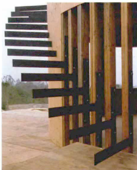
Brackets fit in the wall. The doubled 2x6 studs were laid out on 9 ⅜-in. centers—the run of the stairs at the wall—so that a welded-steel bracket could be bolted to each stud.
