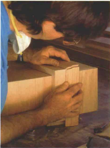
Fitting the colonial stop. The joint between the frieze box's solid-oak lower half and its plywood upper half is covered by a 1x4 oak apron to which is affixed the colonial stop.
