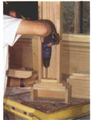
Joining the pilaster to the capital. After building up the capital with two 1-in. oak spacer blocks, the pilaster's plywood end is screwed to the capital. All of the blocks are flush.
