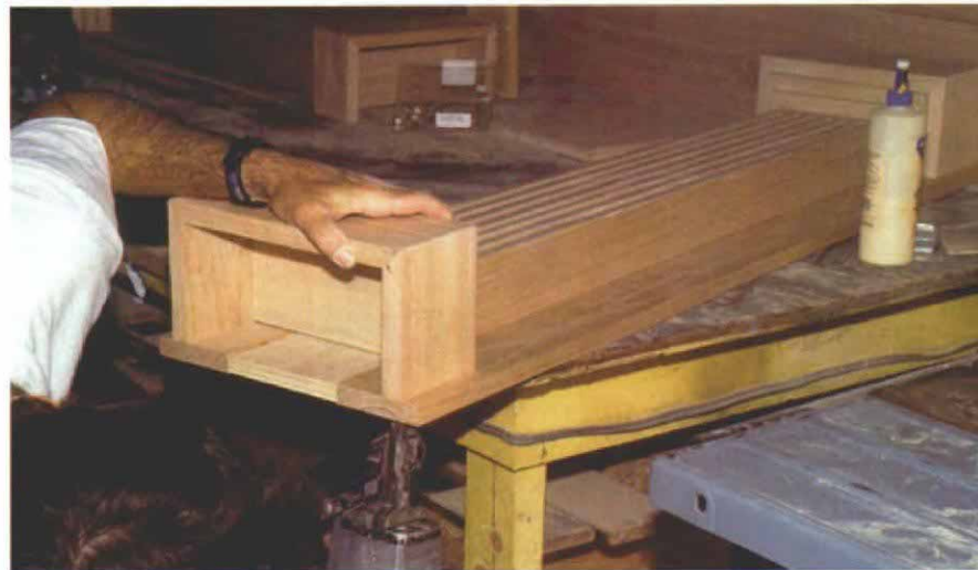
Use plywood where it won't show. Nailed to the pilaster, a backboard eliminates the need to scribe fit the fireplace's marble veneer to the pilaster profile. For economy's sake, the backboard consists of two pieces of solid oak on the exposed ends and plywood in the hidden center, all glued and biscuited together.
