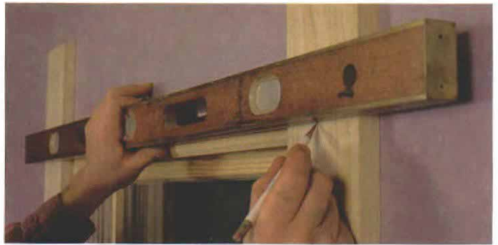
Connect the marks with a straightedge. Using a straightedge to mark the side-casing top cuts will ensure that the head casing fits perfectly. Simply squaring cuts from the marks can result in sloppy joints.
