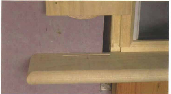
Biscuits register side casings to stool. Common practice is to nail up through the stool into side casings. But biscuits hold better than end-grain nails and won't come out through the exposed surface of the side casing.
