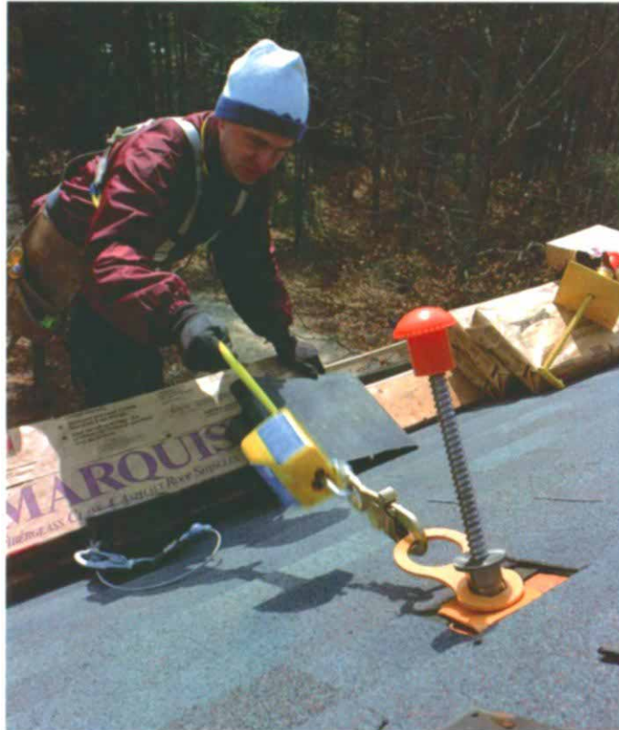
Free to concentrate. A secure roof anchor, a snug body harness and a good lifeline allow this roofer to concentrate on the job at hand.
