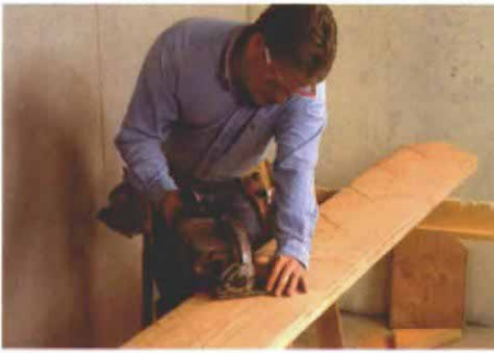
First cuts are made with a circular saw. Overcutting the lines will weaken the stringer, so the initial cuts with a circular saw should never extend beyond the layout lines.
