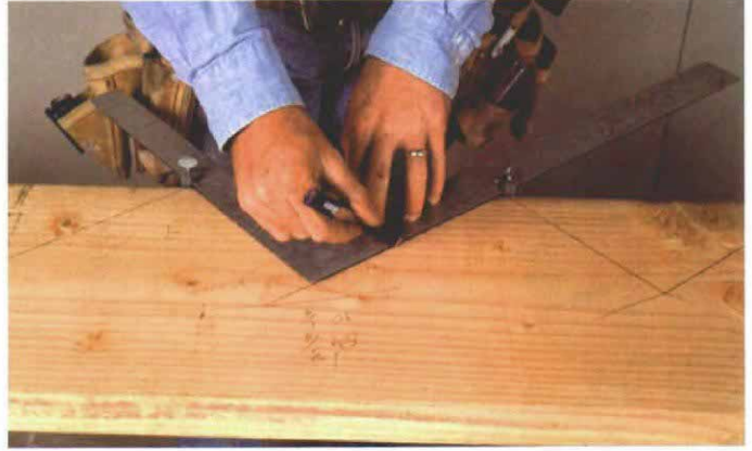
Stair gauges streamline layout. Small clips called stair gauges are attached to the framing square at rise and run measurements to keep the orientation of the framing square the same for each step layout.
