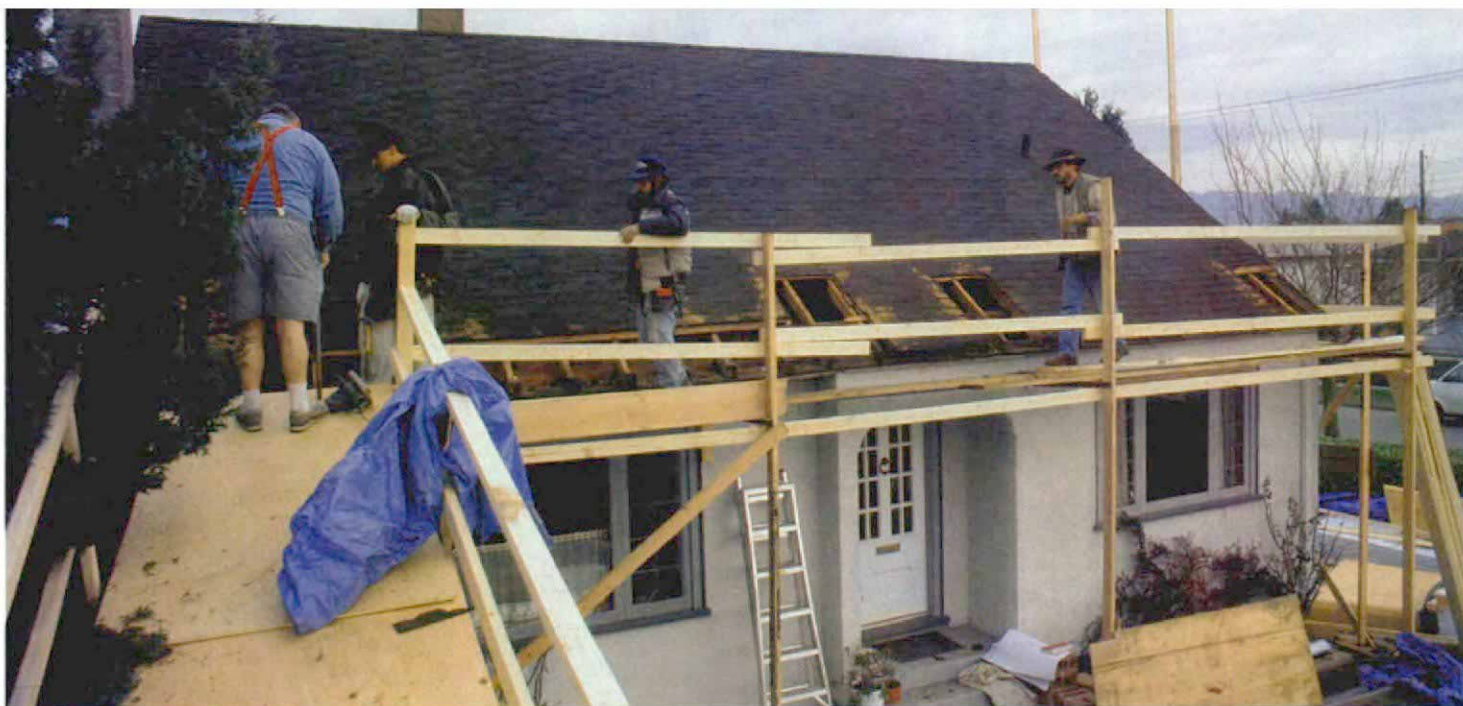
Preparing for the new roof. The crew begins construction of the new roof by excavating post holes in the old roof over the wall plate. On the left, a ramp for removing roof debris leads to a curbside Dumpster.
