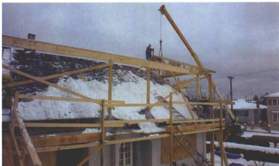
Posts carry a wall beam. Well-braced with diagonal 2x4s, 4x4 posts rise from the holes in the roof to support a doubled 2x10 beam. Note the temporary flashings that are at the base of the posts. At the far end, the wall beam extends beyond the plane of the house to create a staging area for the roof trusses.
