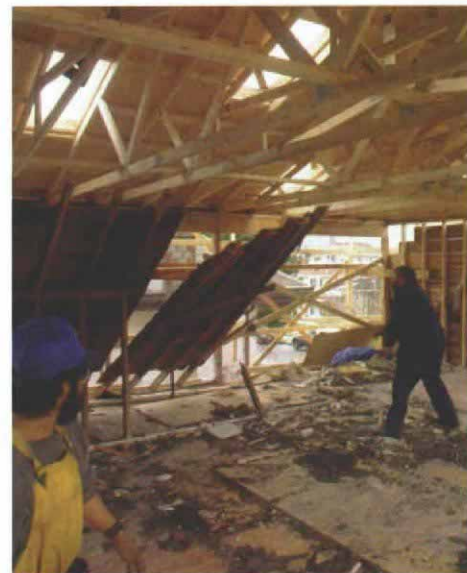
The old roof comes down. With the new roof in place, the old one can come down. Next, the missing studs in the perimeter walls will be installed.
