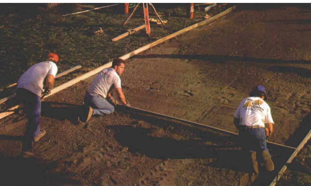
The base layer is graded to the proper height. The laser level in the background is used to set the forms to the correct height. The crew then grades the base to the forms, and the base gets compacted one last time.
