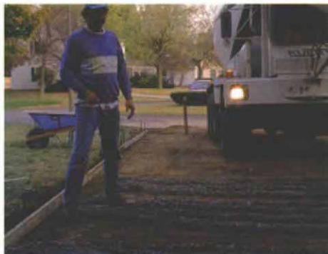
Wire mesh is pulled up on top of a thin layer of concrete. A crew member pulls the wire-mesh reinforcement up to the proper height with a rebar hook. A bead of concrete laid first supports the mesh during placement.
