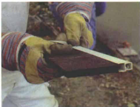
Expansion joints get a plastic cap for installation. Expansion joints act as buffers between driveway sections. After the concrete has cured, the plastic cap is removed, and sealer fills the joint to keep out moisture and light.
