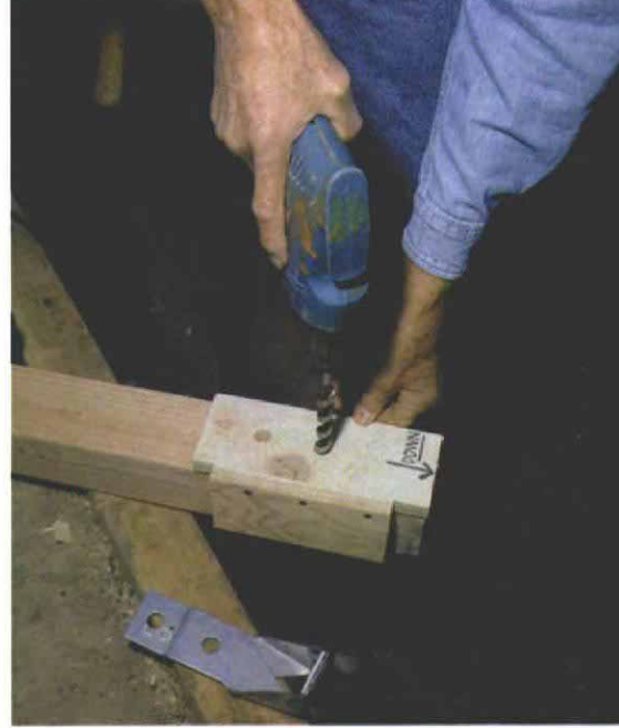
Drilling guide locates bolt holes. A simple template makes fast work of drilling holes for hold-down brackets.
