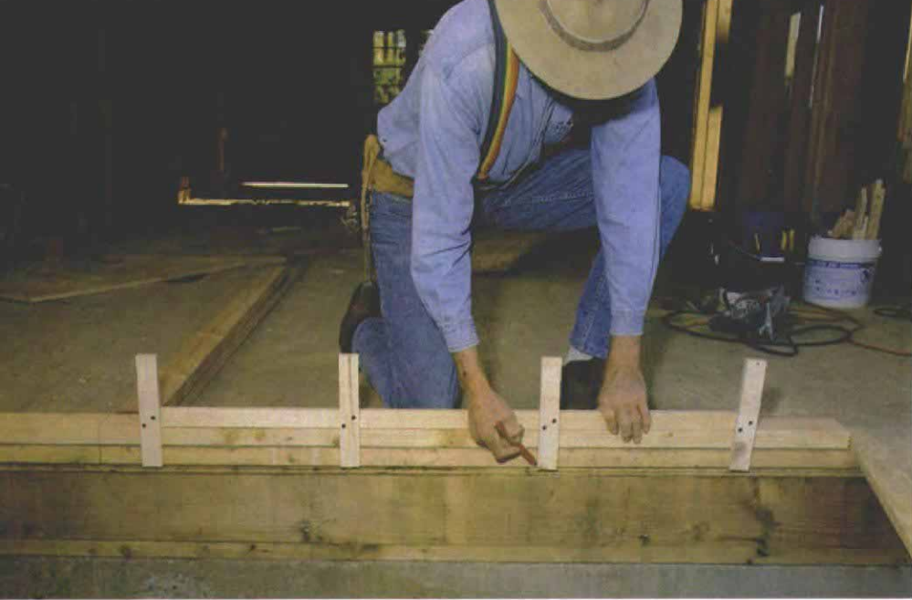
A homemade template speeds stud layout. Using a layout stick to mark stud locations can be faster than measuring 16in. increments with a tape. Metal layout sticks will last longer, but scrap plywood works fine in a pinch.
