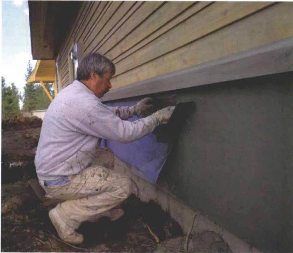
Mesh reinforcing is embedded in the base coat. A thin layer of base coat is applied to the insulation before the fiberglass-reinforcing mesh is rolled onto the wall surface. More base coat is applied over the mesh.
