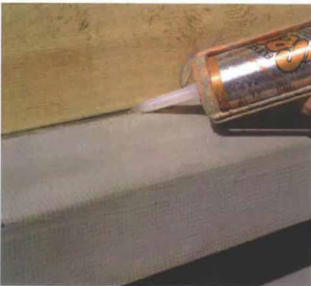
Caulk the base coat, not the finish. Sealant recommended by the manufacturer is applied wherever the EIFS intersects other materials, such as at this strip of molding separating the EIFS from the clapboard siding.
