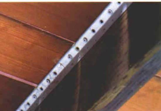
Hidden fasteners attach deck boards. Galvanized-steel angles affixed to the joists provide a flange for screws driven from below.
