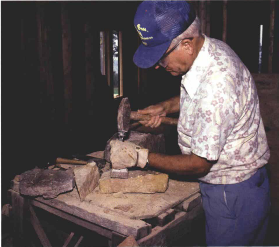
Fine-tuning the stone for a perfect fit. Most stonework requires some chiseling to get the stones to fit correctly. Here the author uses a standard mason's chisel to dress the face of a stone.
