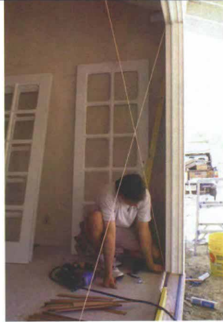
Checking for cross-legged jambs. Strings stretched from corner to corner will touch in the middle if jambs are in precisely the same plane, which ensures the door slides smoothly.
