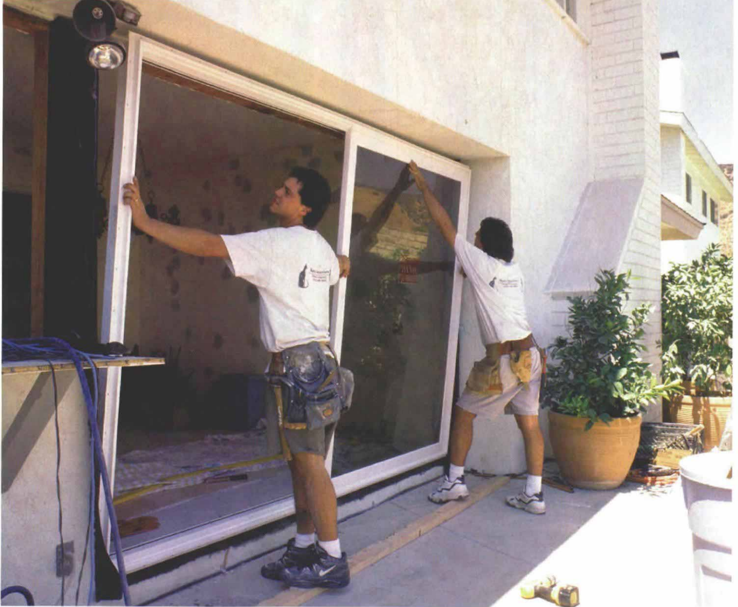
Slider frame is bedded in caulk. Caulking is applied around the framed opening, and the nailing flanges on the side jambs are pressed into the caulk and fastened temporarily until the jambs are plumbed.
