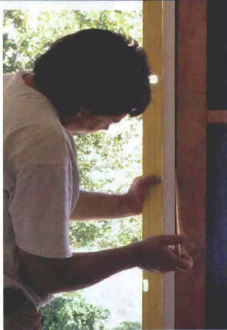
Shims bring the jamb out to the level. After the sill is leveled and the jambs are plumbed top to bottom, shims are inserted behind the jamb until the jamb touches the level.
