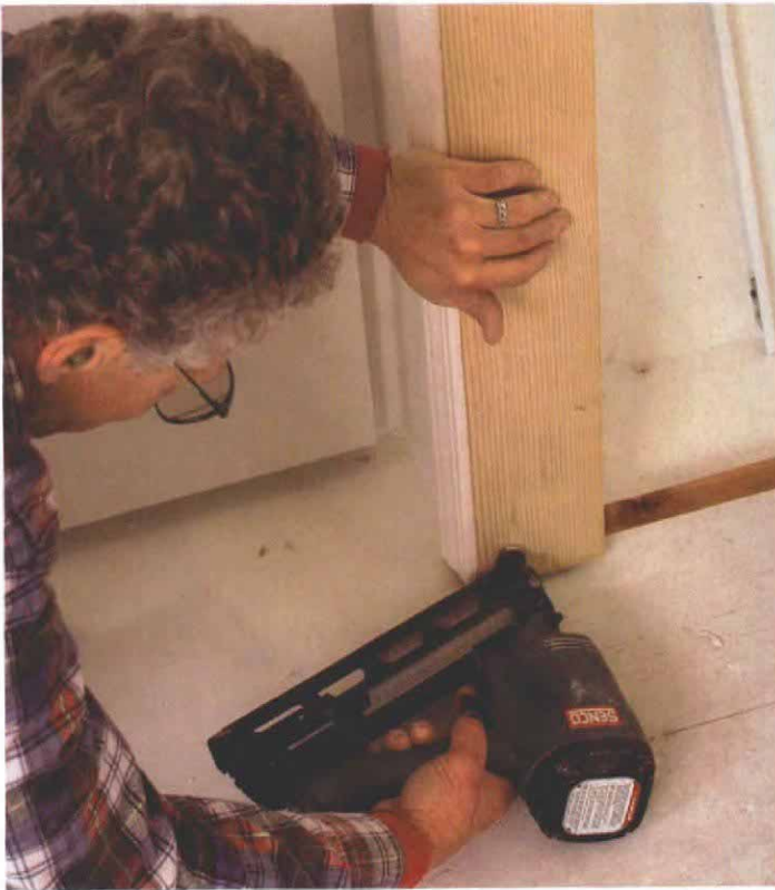
8. Shim the jamb, and nail it home. Once the jamb has been plumbed, it can be permanently affixed to the trimmer. Britton uses a 15-ga. nailer, driving the fasteners through shims to keep the jamb from deflecting toward the framing as the nails slam home.
