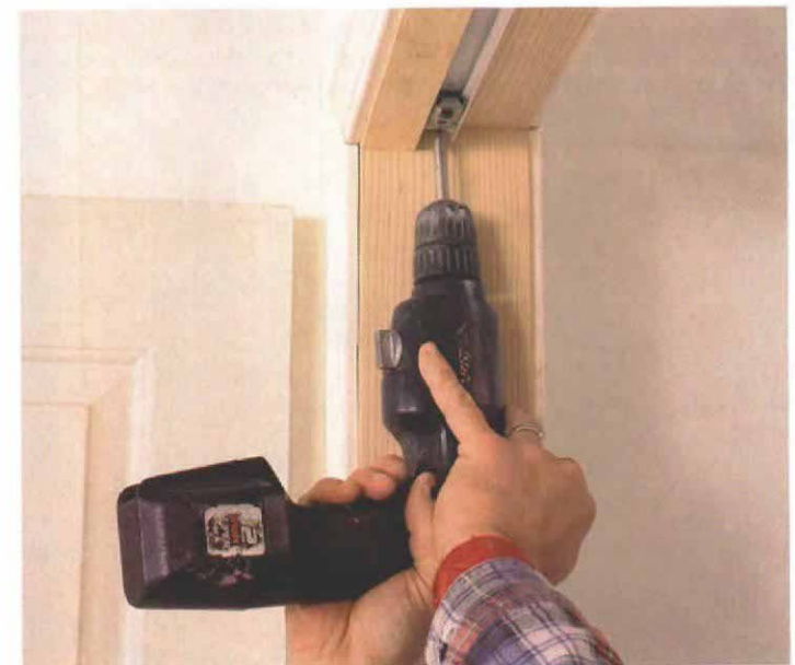
11. Screw the track to the head jamb. The door track fits flush against the 1x2 nailed to the inside of the head jamb. If the screws reach the header, be sure to shim the jamb to keep it from deflecting.
