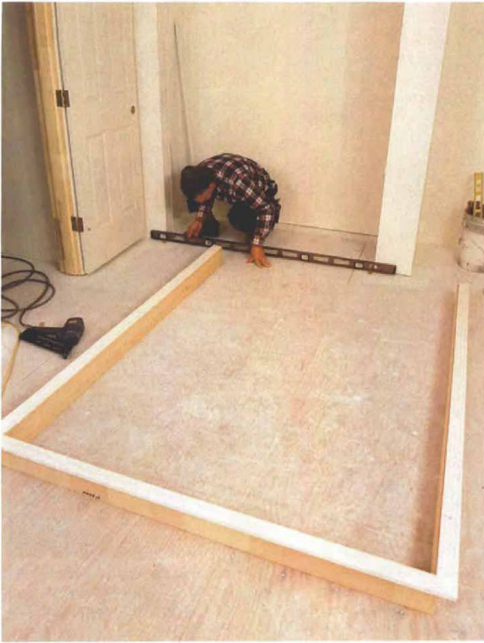
4. Shims elevate the jambs. With a spirit level long enough to span the rough opening, the author assesses the floor for level and places shims accordingly next to the trimmer studs. The shims, which are at least \frac{3}{8} in. thick, lift the jambs enough to accommodate the carpet.
