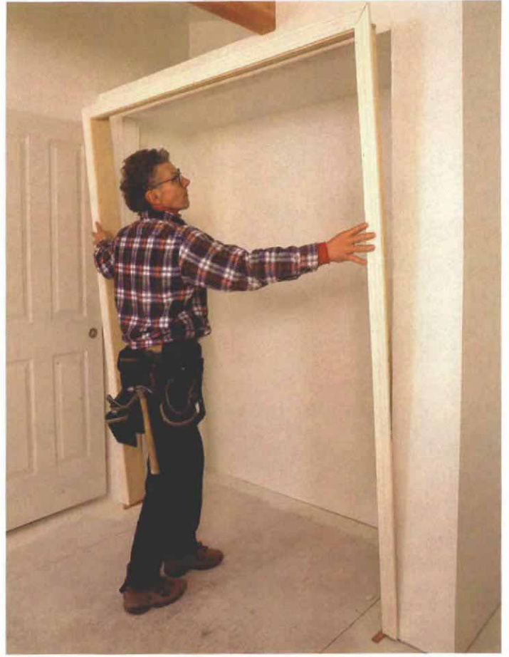
5. Lift the pretrimmed jamb into its opening. With the bottoms of the side jambs sitting on their shims to ensure a level head jamb, Britton slides the jamb assembly into the rough opening. Affixing it to the rough-opening frame starts from the top down.
