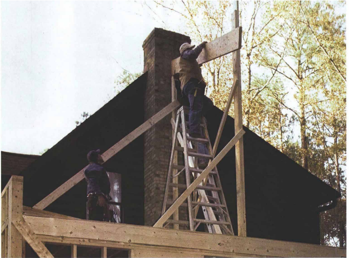
Setting the ridge. Temporary posts are set up to hold the ridge at the right height. The posts are braced 2x4s with a 2x4 scrap nailed to the top that rises 10 in. above the top of the post. The ridge is set on top of the post and nailed to the scrap of wood.
