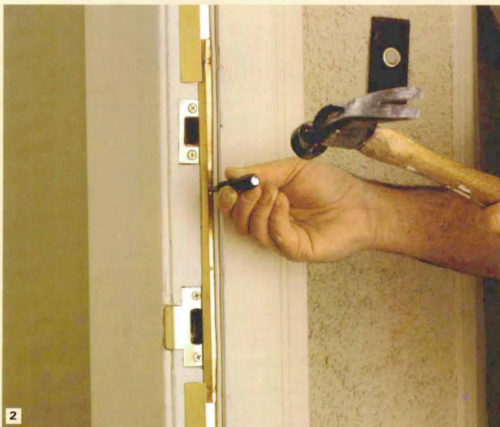
Leave room for the lockset. Strike plates for a dead bolt and latch require narrow V-bronze. Be sure to cut it long for plenty of overlap, and set the nails carefully to avoid marring the bright surface.
