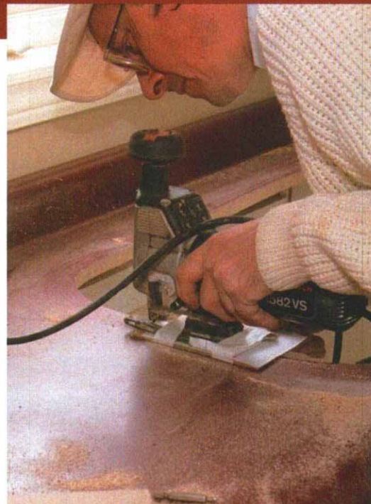
The sink is the last step. With the template supplied by the sink manufacturer, cut the sink opening in the countertop. To prevent an accidental scratch, the author attaches cardboard to the base of his jigsaw for cutting the hole for the sink.
