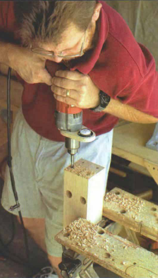
Bubble level keeps the drill straight. After drilling access holes in the newel, the author clamps the post plumb and drills four bolt holes that must be true. The bubble level's plywood base fits tightly onto the drill's motor housing.
