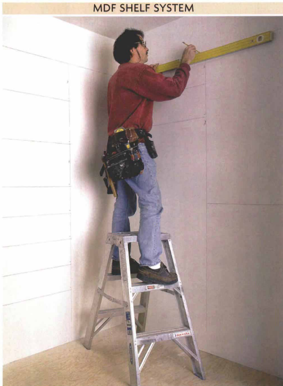
MDF shelving has to be laid out on the wall. Because MDF shelving is supported on permanently mounted cleats, the entire layout is done on the unfinished closet walls.
