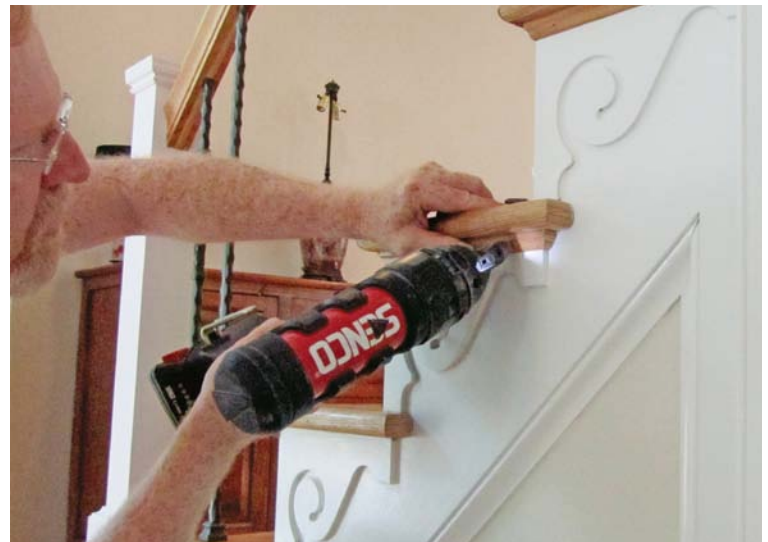
Tread molding is the final touch. Wrapping around the brackets and ending with a glued-on return, this prefinished molding is attached with 18-ga. brads.
