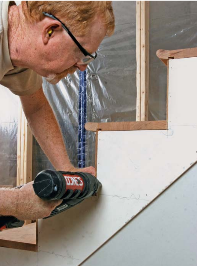
Fasten the skirtboards. The riser miters extend past the skirts to accommodate the decorative brackets.
