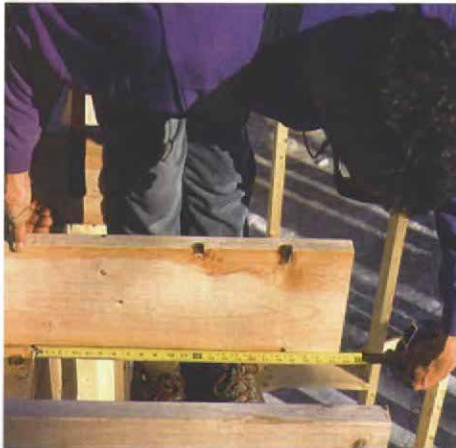
Setting the overhang. With a 2-ft. cantilever, the longest joists overhang 22½ in. The joists are then tacked in place.
