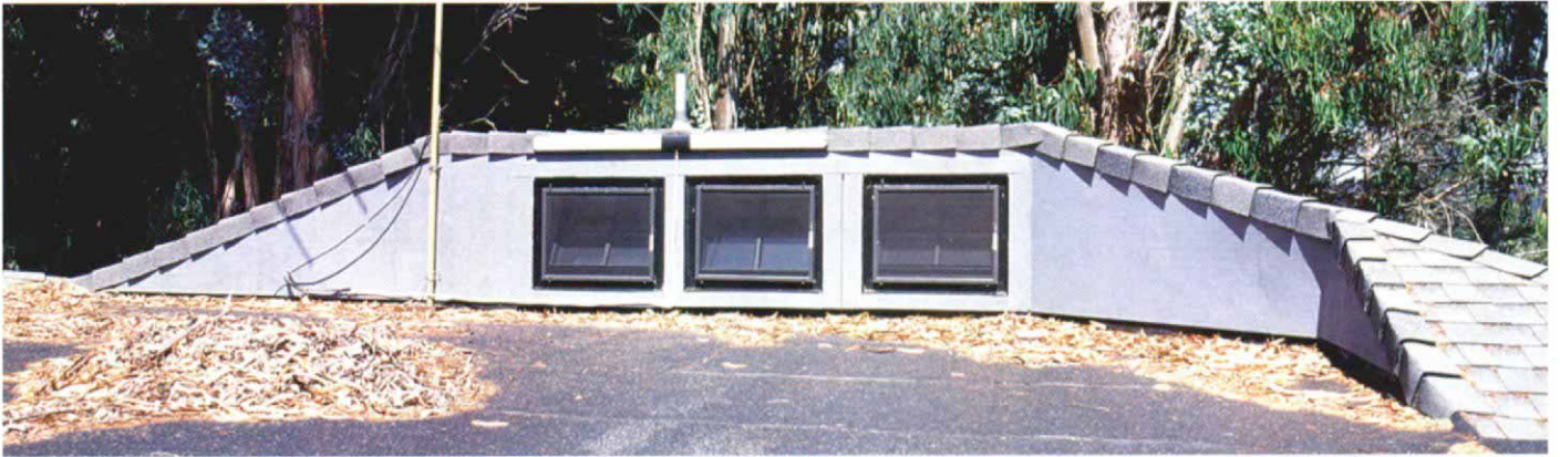
The drama is on the inside. Hidden behind a hip roof that ties a flat-roofed 1960s addition into the roof line of the rest of the house, clerestory windows deliver southeastern light to the new master suite. Photo taken from roof level at C on floor plan.
