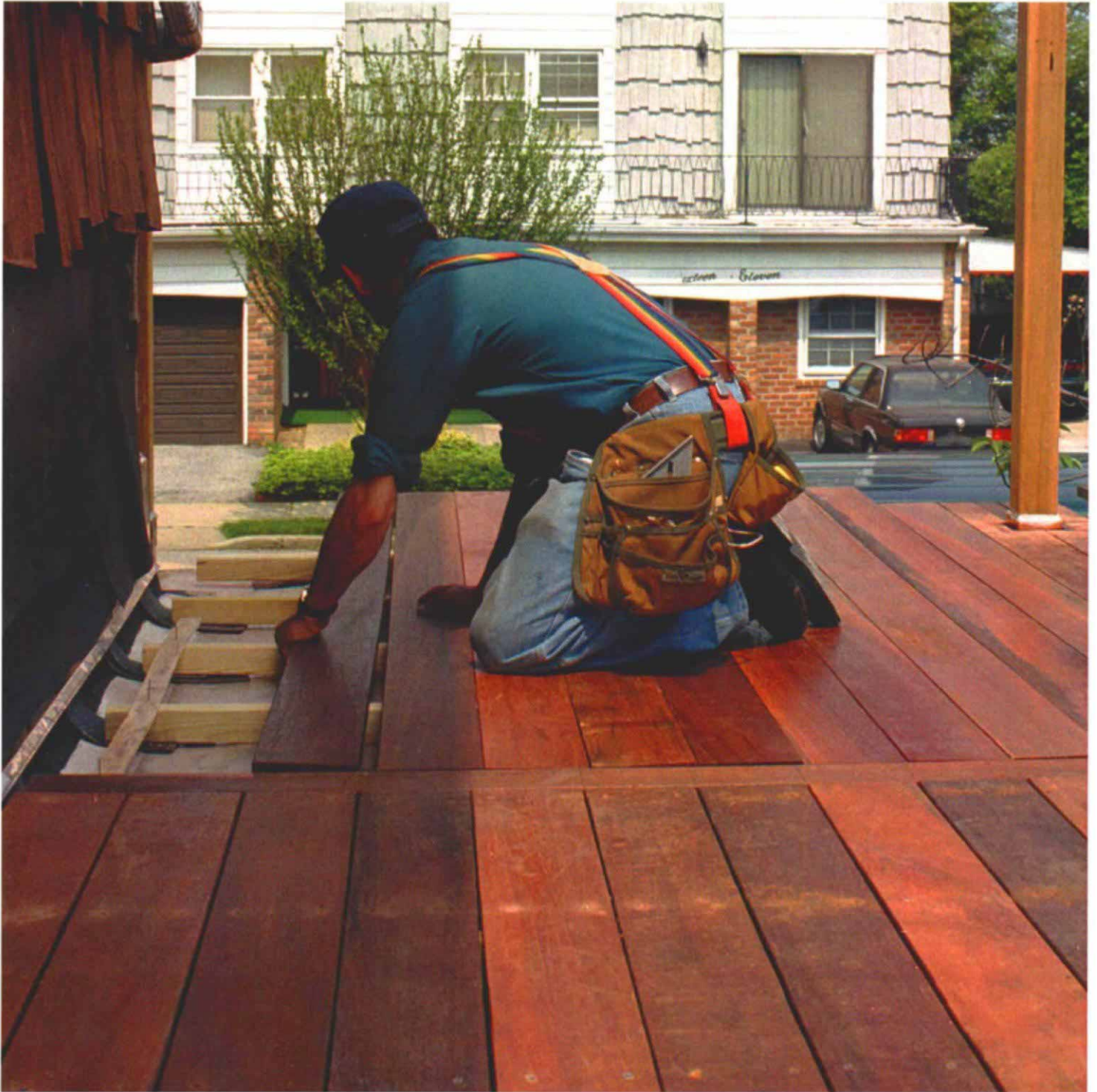
Modular deck framing allows access to the roof. The deck was framed in sections to make future access to the membrane easier. Small pads of bituminous membrane keep the pressure-treated frame from damaging the rubber skin of the roof.
