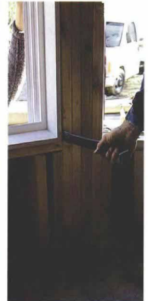
Pop in the window. As you would set a wood window, the bottom of a vinyl unit is rested on the rough sill; then the unit is pulled into the rough opening. A carefully wielded pry bar is used to center the window.
