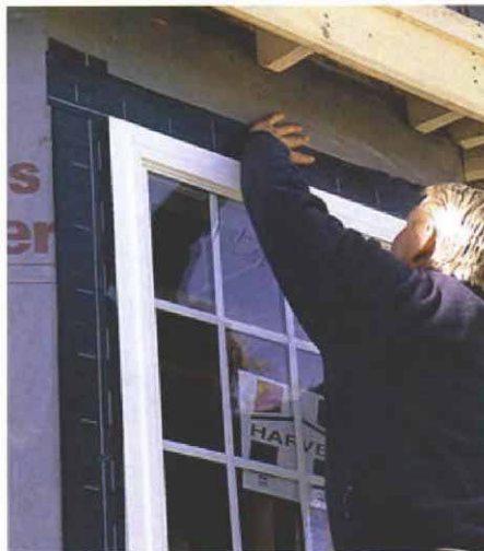
Roofing nails hold in vinyl windows. Here's about the only difference in installation: Vinyl is easily cracked by an errant hammer blow, particularly in the cold. Once the window is in, self-adhering flashing tape seals out water.
