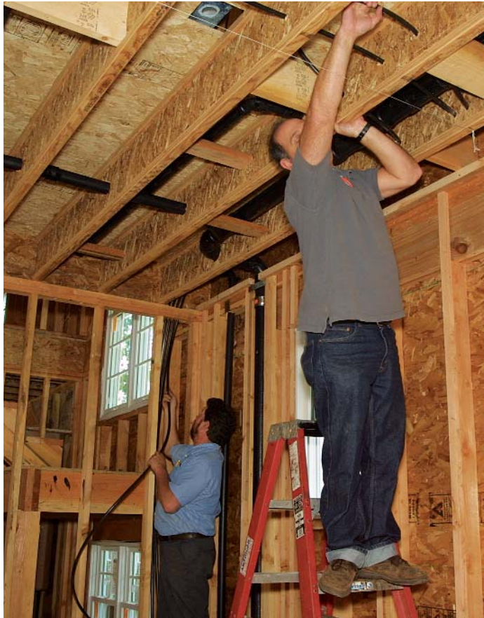
An extra pair of hands prevents kinks. Although PEX can be pulled like wire, it can kink or even be punctured. It's a good idea to have help when pulling the flexible tubing.
