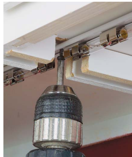
You need short screws and a little screw-driver. An adhesive strip holds the track in place while the track is fastened with short screws. A terminal block at the end has small screw-down connectors for the wire.
