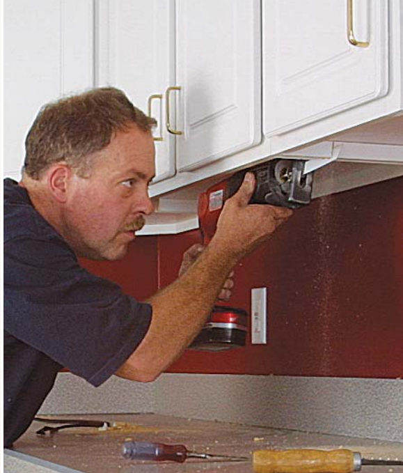
Customizing a stock cabinet. A 1-in.-wide channel cut in the bottom of the cabinet sides allows for a continuous track. Cutting the channel 2 in. back from the front of the cabinet keeps the track concealed behind the bottom lip of the cabinet and will shine light directly on the work zone in the middle of the countertop.
