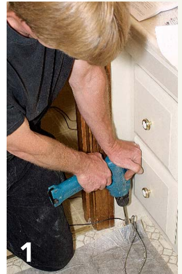
1 Locate the electrical feed. With the heat mat temporarily in place, the electrician drills in an inconspicuous spot to run wiring for the electrical feed and thermostat control.
