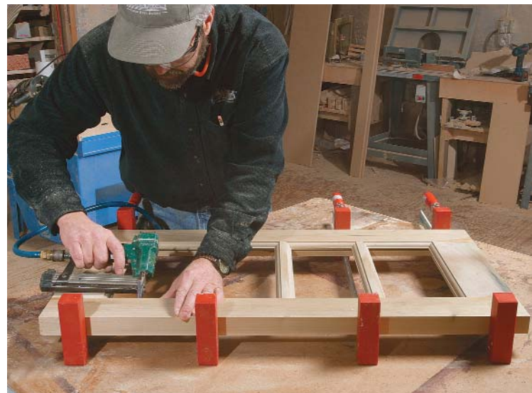
Fill in the blanks. While the glue dries, the last pieces of the stop go in along the rail. After the transom is installed and the glass panes are set, additional stops are applied to the other side.
