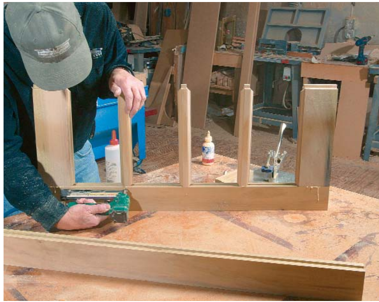
Headless pins speed assembly. After the stop has been applied to the stiles and muntins, headless pins help to hold the pieces in position until the window is clamped.
