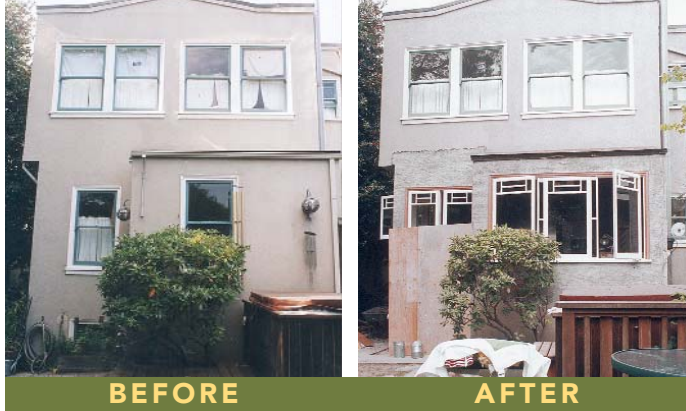
New windows unify the look. Because the new windows take up more wall space than the old ones, extensive structural reinforcement had to take place before installation. Photos taken at B on floor plan.
