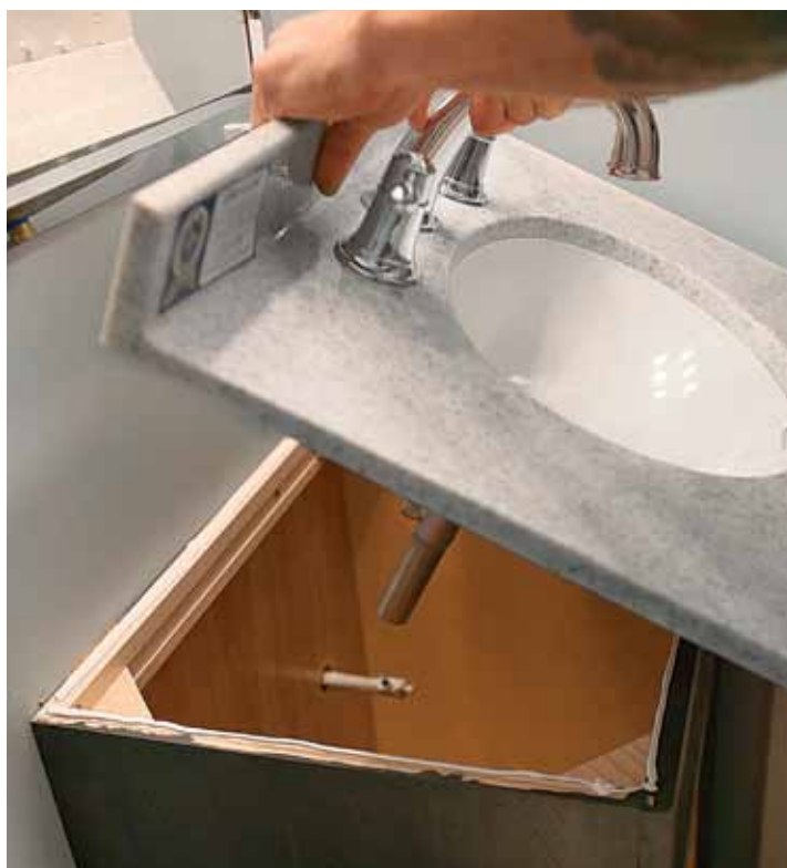
Wet set. After confirming that the countertop scribe fits the wall, apply adhesive caulk to the inside edge of the cabinet to avoid visible squeeze out as the top is set and taped into place to cure.
