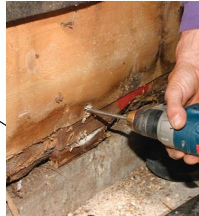
Drilling a pilot hole through the rim joist makes it easier for me to start the cut with a reciprocating saw.
