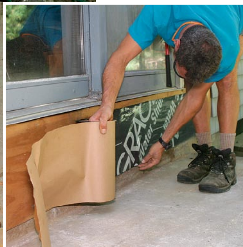
Peel-and-stick shingle underlayment protects areas vulnerable to water damage. Housewrap will become a second line of defense behind the siding.
