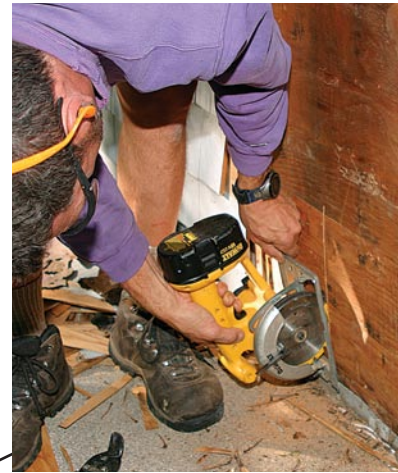
A circular saw and an accurate depth of cut make it easy to remove the plywood sheathing and expose the rotten section of rim joist.
