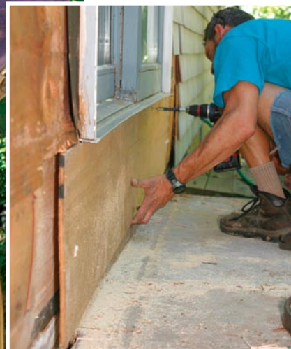
Half-inch exterior-grade plywood is cut to fit over the repaired sections of mudsill and rim joist, then fastened in place with screws.
