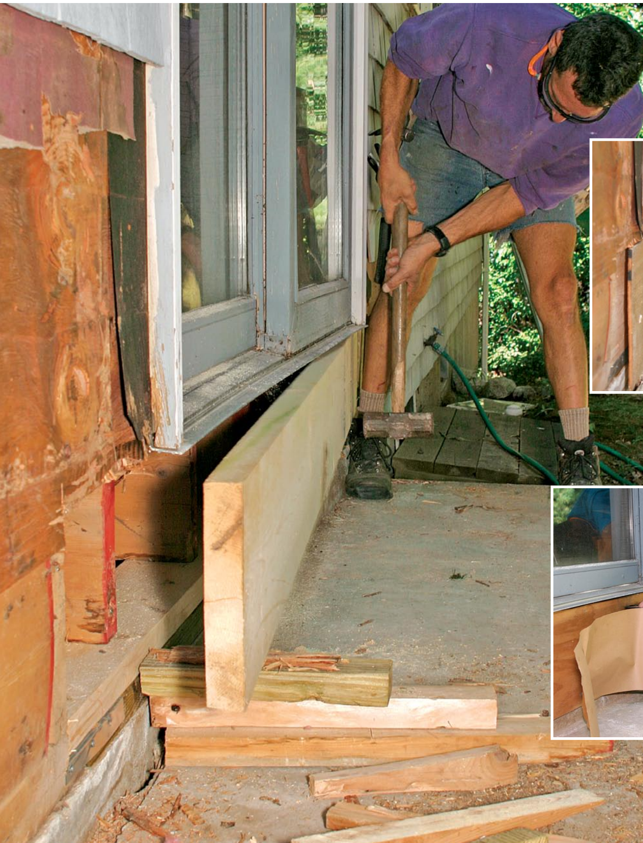
When working alone, I use scraps of lumber to support the opposite end of the rim joist at the proper height while it's hammered into place.
