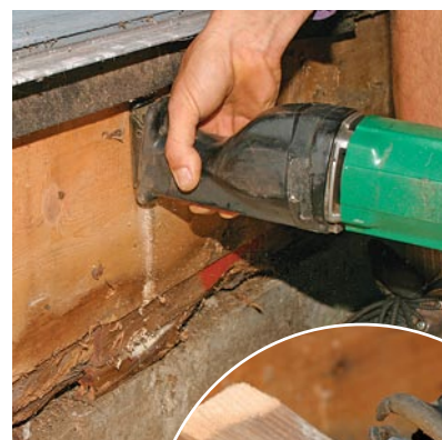
I snap off the tip of a reciprocating-saw blade so that the remaining saw stroke penetrates only to the depth of the rim joist. This helps to prevent damage to hidden utilities running behind the joist.
