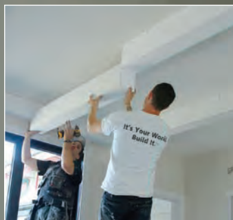
Fill in the grid. Once the perimeter and the long interior beams are installed, shorter pieces are cut and fit in between. A compact laser projects the layout marks across the entire ceiling so that the beams are placed straight.
