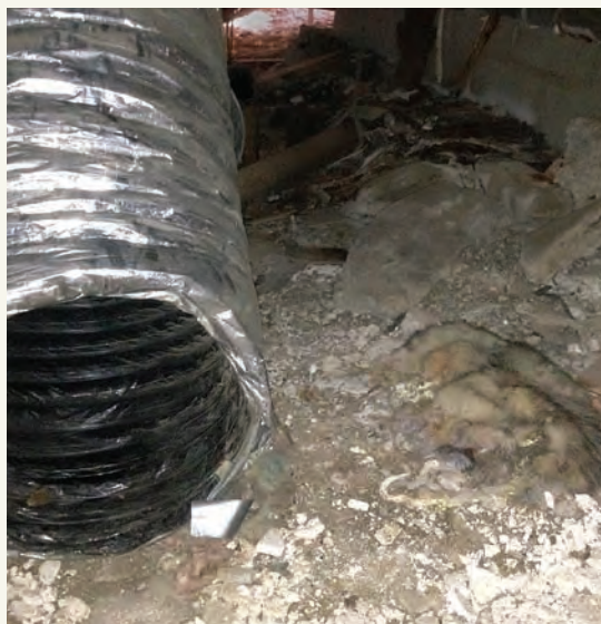
It's what's in the air that matters. A disconnected return duct in most any crawlspace is bad news. In addition to sucking in mold and pesticide residue, this one spices the air with the aroma of dead possum.
