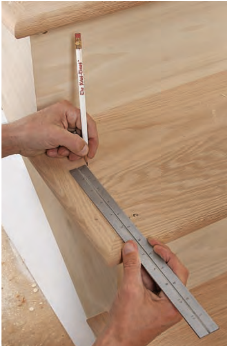
Set the spacing. Locate the first baluster so that its face aligns vertically with the face of the riser below it. Set the second baluster half the distance of the stair run behind the first.
