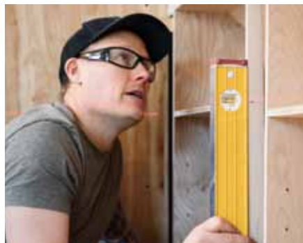
Laser level and plumb. Set to the height of the cabinet's fixed shelves, a laser line is used to ensure each carcass is at a level height with the adjacent units. Young uses a level to check that each unit is installed plumb.
