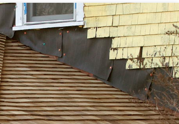
An invasive reroof. A fair amount of reshingling on the sidewalls is necessary to flash this new roof correctly. This problem could have been avoided with counterflashing.
