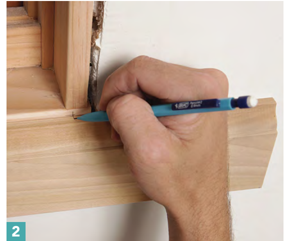
2 Mark in place. Transfer the marked reveals to the stock, and label each piece to indicate its place on the opening—top, bottom, left, and right—and the opening it belongs to.
