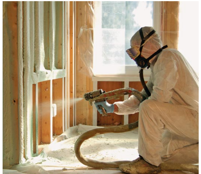
Proper prep yields the best installation. While spray foam is installed by a pro, it's your responsibility to prep the site. Masking windows, electrical boxes, and even floors is important if you want the foam contained to wall, roof, and floor cavities. Anyone on site during the installation should be outfitted for optimum protection.
