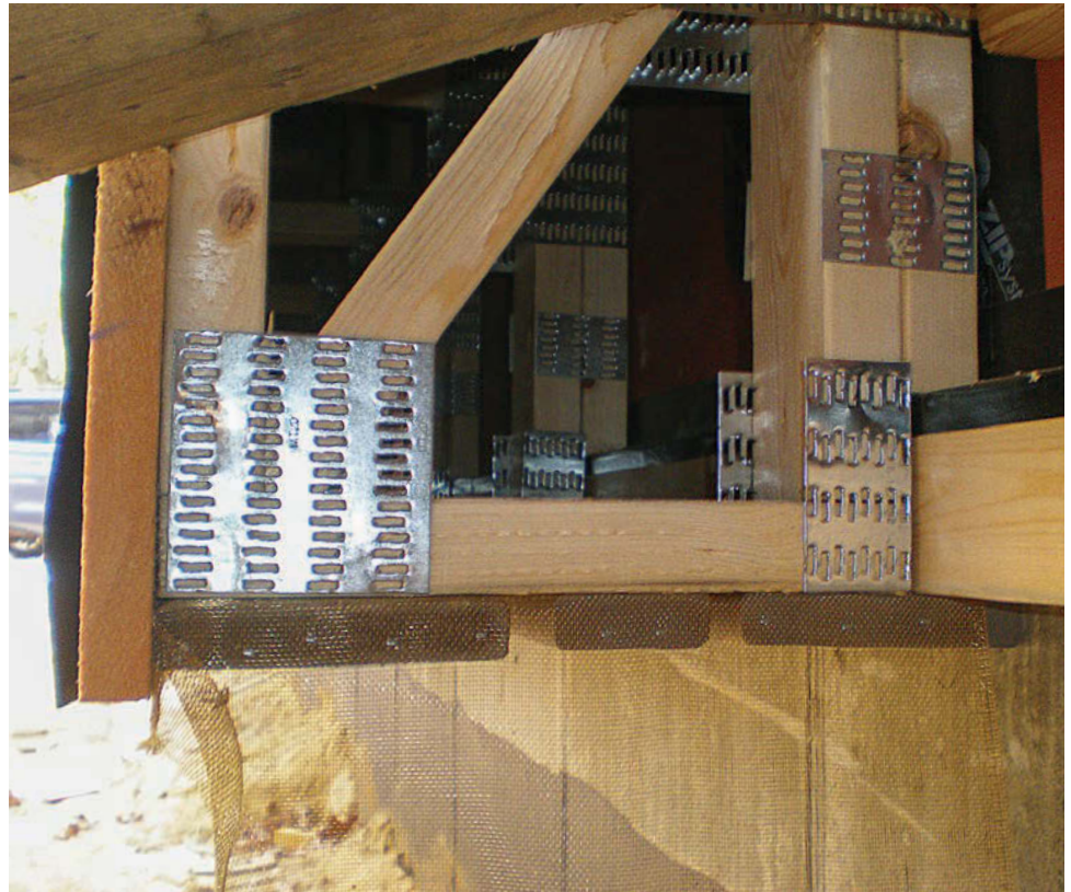
BUTTON UP THE BOTTOM Larsen trusses sometimes sit atop the foundation or the foundation insulation, and sometimes hang outside of the foundation. In any case, you'll need to be able to keep insulation in and critters out. On this project, a combination of insect screen and synthetic deck boards get the job done.
