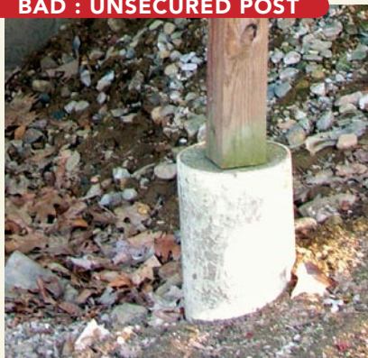
BAD : UNSECURED POST
