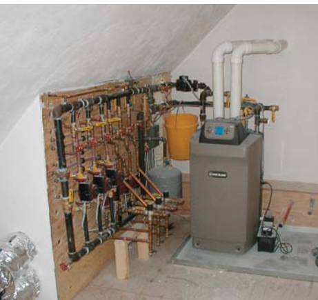
Radiant heat is fueled by a 98.6% efficient Weil-McLain modulating gas boiler ( www.weil-mclain.com ). Cast-iron piping is used wherever possible to limit PVC use.
