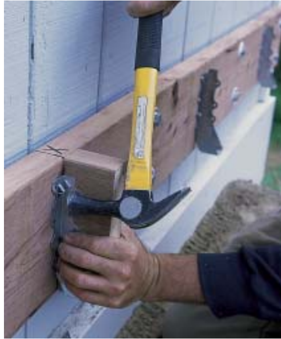
Here a scrap of joist is used to help set the hanger height and keep the side flanges the correct distance apart. Attach the hangers with 1½-in. long galvanized nails made specifically for metal connectors.
