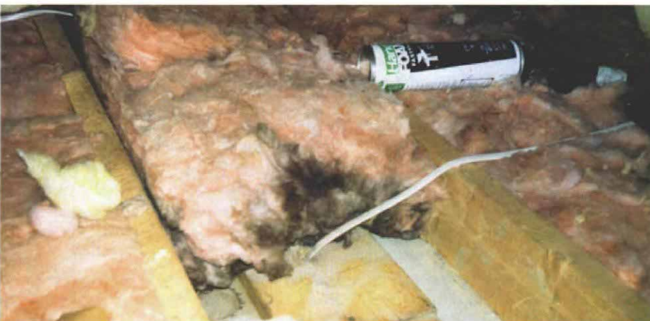
Dirty fiberglass signals an air leak. As warm air pours through penetrations in the ceiling, dirt is filtered out by fiberglass batts, but the heated air goes into the attic. Holes for wiring should be filled with expanding-polyurethane foam to stop the loss of this air.
