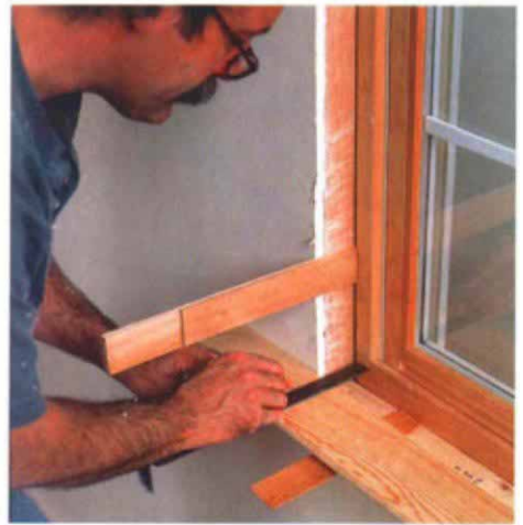
Shims support the stool for layout. The author marks the notch cut on the stool, then measures between it and the window to lay out the rip cut for the horn.
