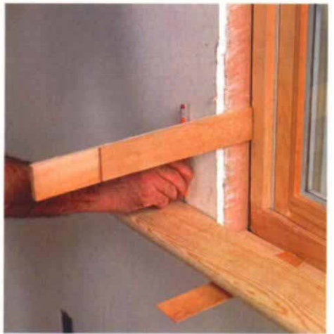
Scribing the stool to the wall. Because the wall is rarely parallel to the stool, this mark, not the edge of the stool, is the baseline for laying out the horn's rip cut.
