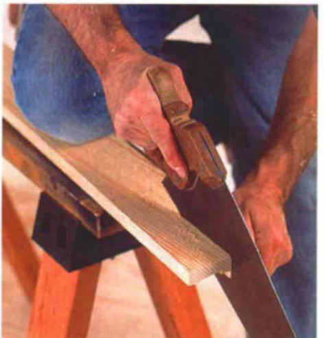
Notching the stool. Although he uses a miter saw to make the crosscut, the author prefers a handsaw for the rip.
